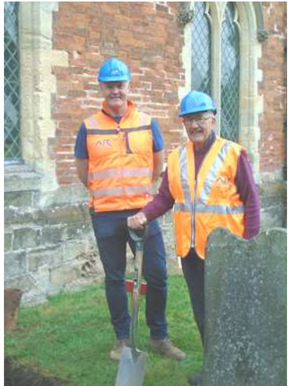
Bill Sharp, PCC Chair, showing Richard Dolman of AR Demolition his prowess with a spade
